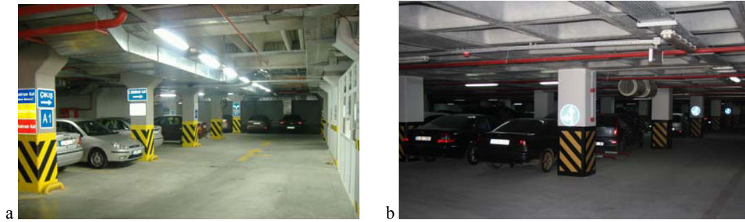
Fig. 1. Underground multi-storey car parks with, (a) with ductwork type ventilation; (b) with jetfan type ventilation.
