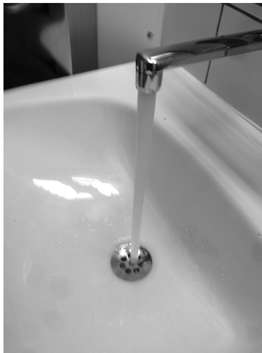
Figure 1. A standard sink in the hospital where water is directed straight into the sink drain.
