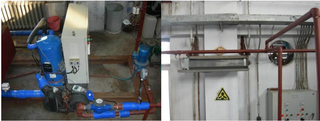
Fig. 2. pictures of heat pump and fan coil in the Lab
