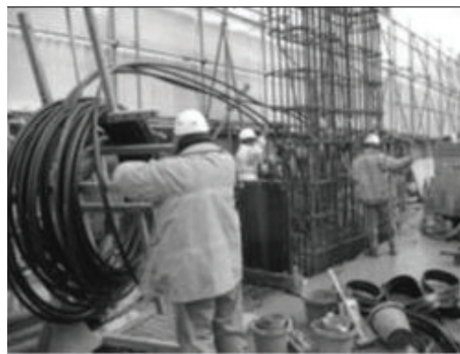
Figure 4: Installation of wall panels & ground loops in wall panel, with permission GI Energy
