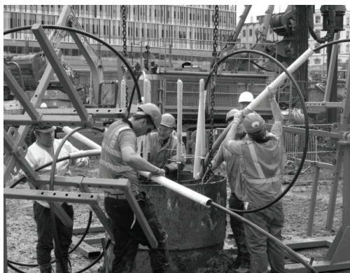
Figure 3: Protection of ground loops at pile head prior to concreting, with permission Cementation Skanska Ltd.
