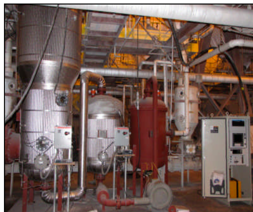
Figure 4: Flue Gas CO 2 Capture and Mineralize Pilot Process. (from right to left: Horiba flue gas analyzer, flue gas inlet, MDR, blower, humidifier, FBR).
