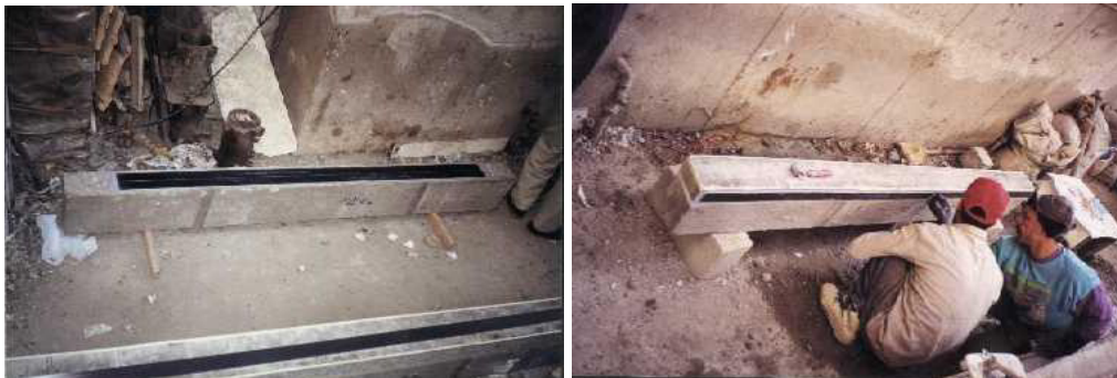
Figure 5. Application of CFRP strips on the bottom and sides of concrete beams
