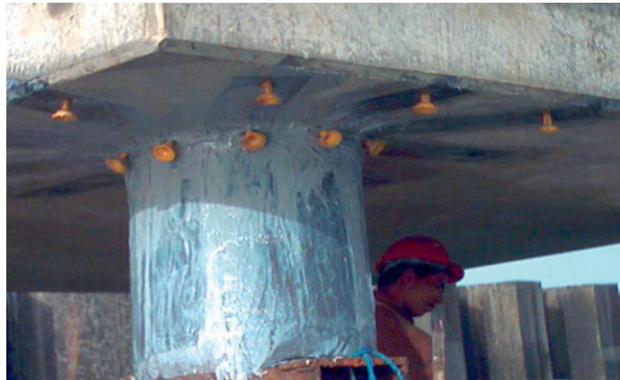
Figure 27. Locations of CFRP anchors
