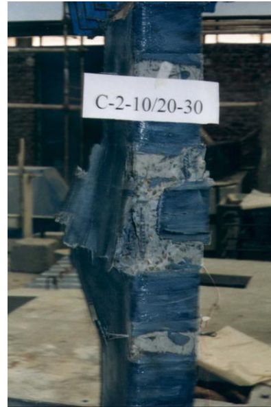
Figure 2. Failure of a rectangular column subjected to axial load
