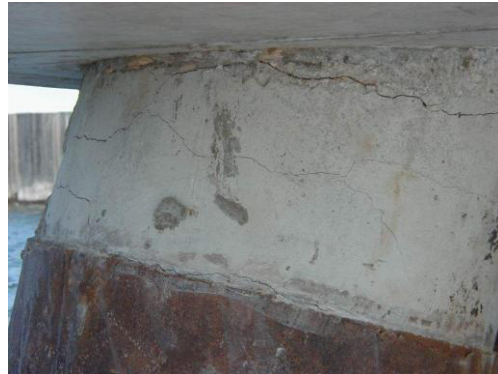
Figure 24. Large widths flexural cracks
