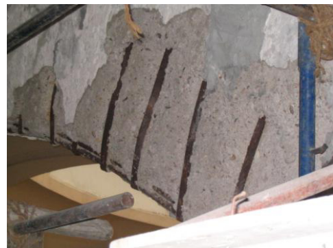
Figure 13. Corrosion of the steel reinforcement
