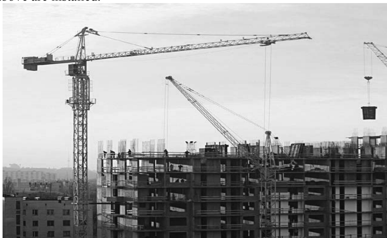
Figure 8: Lack of firefighting provisions in buildings under construction
