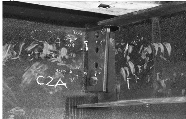
Figure 5: Fracture of connection during cooling, Cardington fire test (Newman et al 2006)
