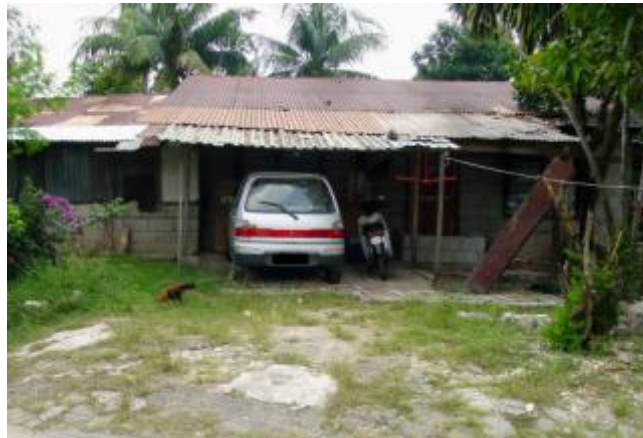
Fig. 1. An example of structural adaptation depicting a house with concrete lower wall
