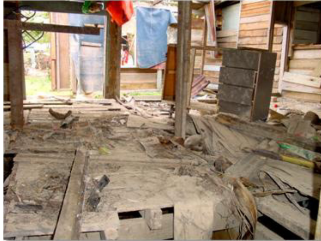
Fig. 2. A flood-damaged house whose owner has moved out of the study area
