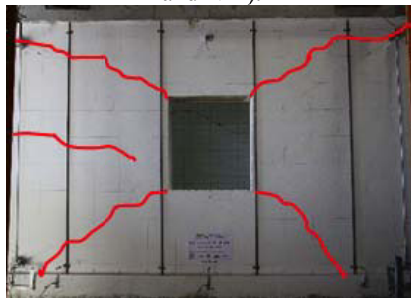
Fig. – Final damage state.
