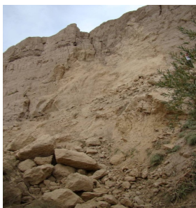
Fig.16 Collapse of cliff face in the east of northern tableland due to impact of seismic load (without conservation).
