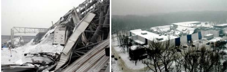
Fig. 1. Exhibition hall in Katowice after catastrophe, [10].
