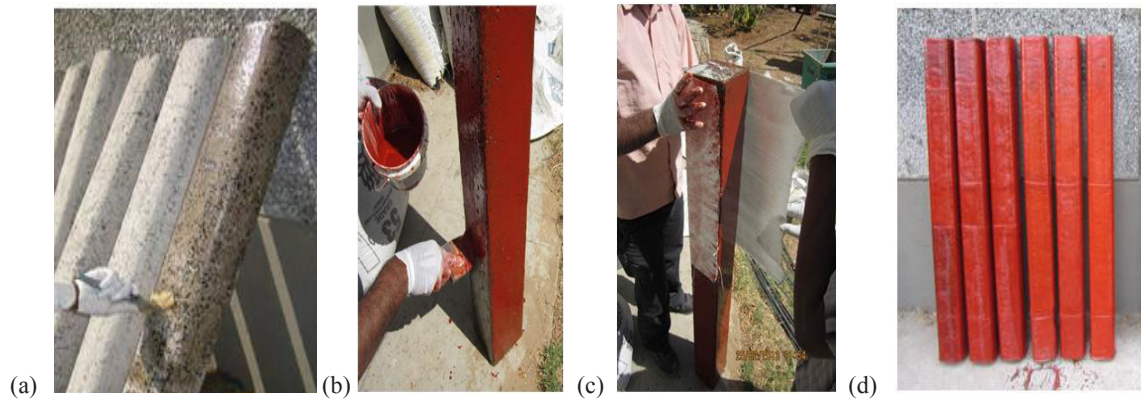
Fig. 4. (a) Application of Primer, (b) Application of saturant, (c) Application of GFRP sheet and (d) After application of GFRP sheet and saturant
