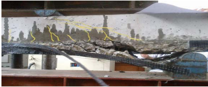
Fig. 5: Shear Failure of beam with de-bonding of CFRP along with concrete
