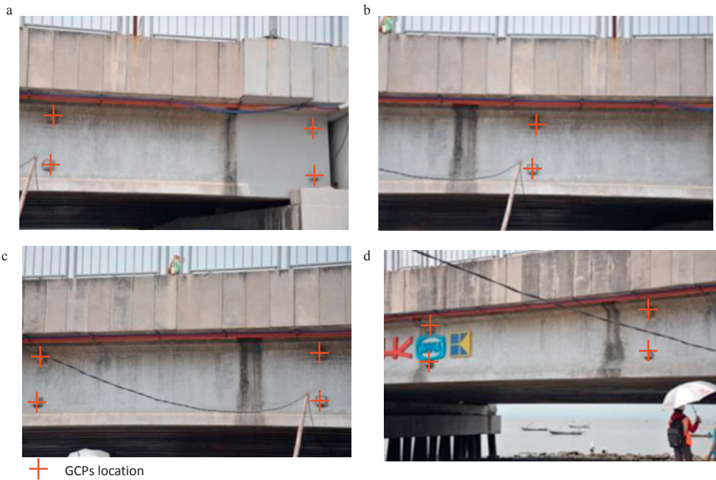
Fig.4. Captured images overlapping one another of bridge spans in Surabaya side with distribution of GCPs (a). first image; (b). second image; (c). third image; (d). fourth image
