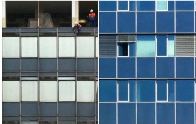
Figure 1: Retrofit of the campus building (2013). Left: dismantling of original curtain wall from 1971 (overall U-value approx. 3.0 \text{ W}/(\text{m}^2\text{K}) ). Right: New curtain wall, triple glazing, venetian blinds motor controlled, overall U-value 0.7 \text{ W}/(\text{m}^2\text{K}) , fenestration ratio 60 %
