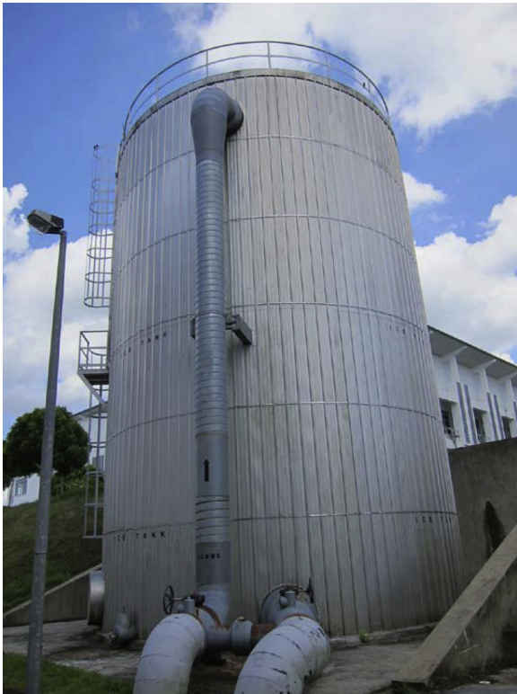
Fig. 3. The ice thermal storage (capacity rated at 7000 RTh).
