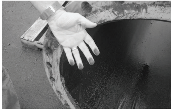
Fig. 1. Evidence of material regeneration around full pipe circumference in 800 mm main 12 months after invasive cleaning
