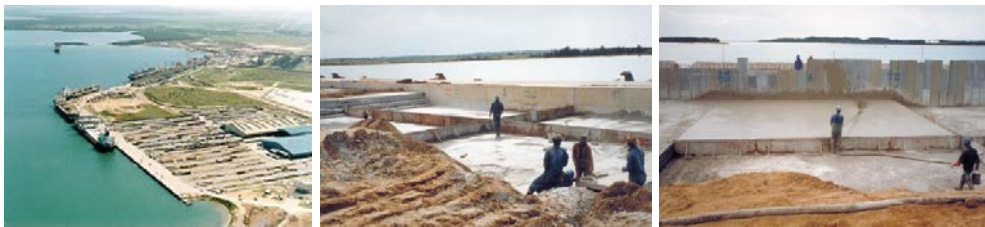
Fig. 3. South Africa's busiest port, foam concrete being placed in 600 mm deep fills, [7].
