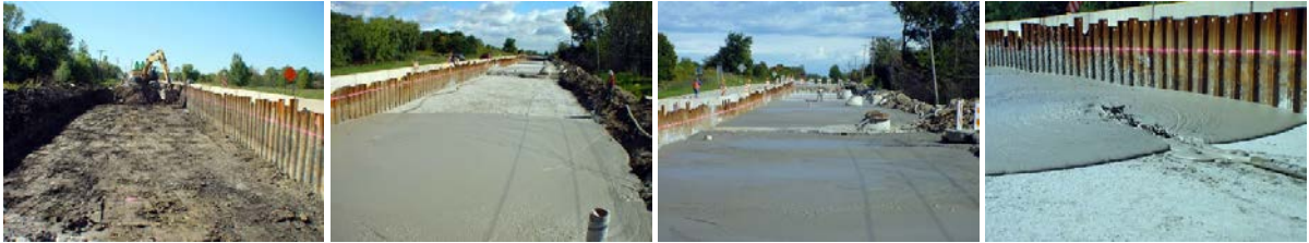
Fig. 2. Views of a typical “Two-stage” road fill project where steel sheeting is installed down the centreline of the roadway to support live traffic while excavation, placement of foam concrete, and pavement construction can be performed in the first stage, [6].
