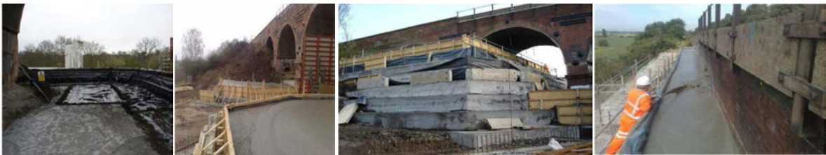
Fig. 1. Views of preparation of the underlay, a poured layer of foam concrete, the pyramidal formwork and application of the last layer of foam concrete, [5].
