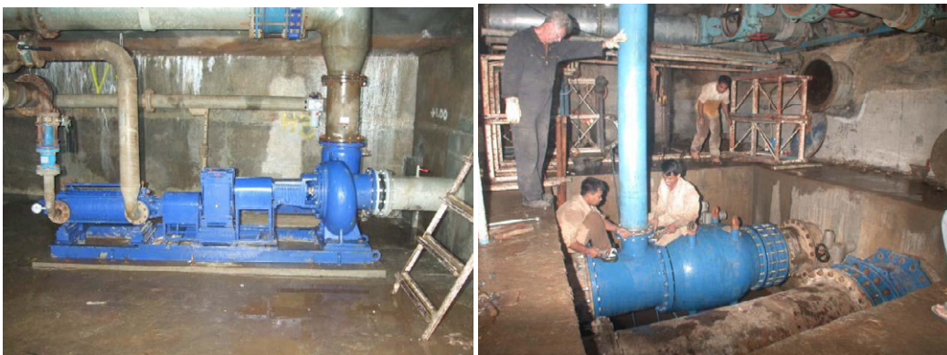
Figure 7. First installed KSB-Module (left), Installation of VAG-valves at flood relief lines (right)
