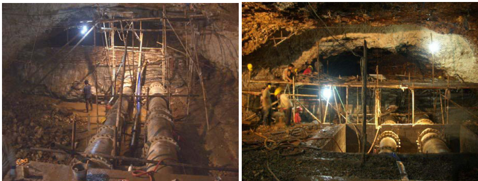
Figure 4. Flood relief lines (left) and status of the construction site in November 2005 (right)
