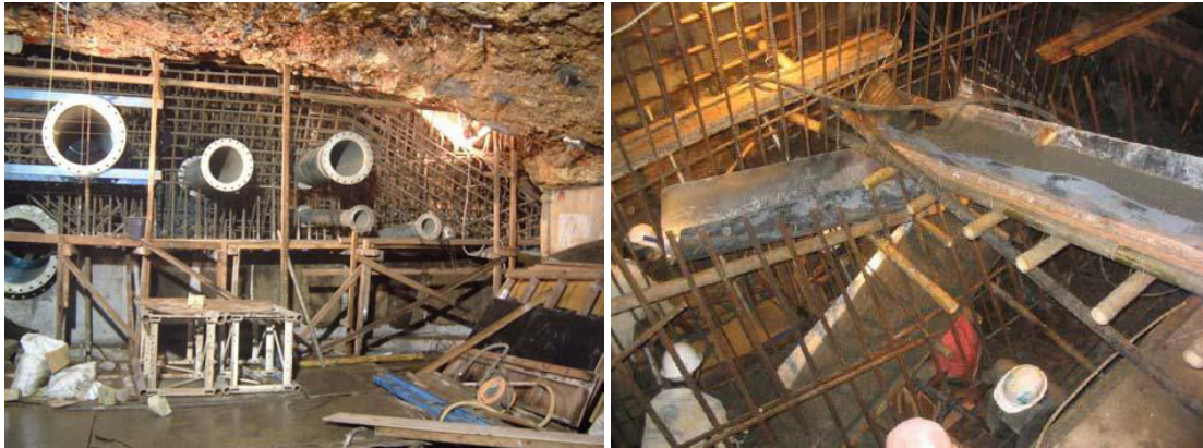
Figure 6. Construction of the barrage with wall pipes (left), transportation of concrete in the cave (right)
