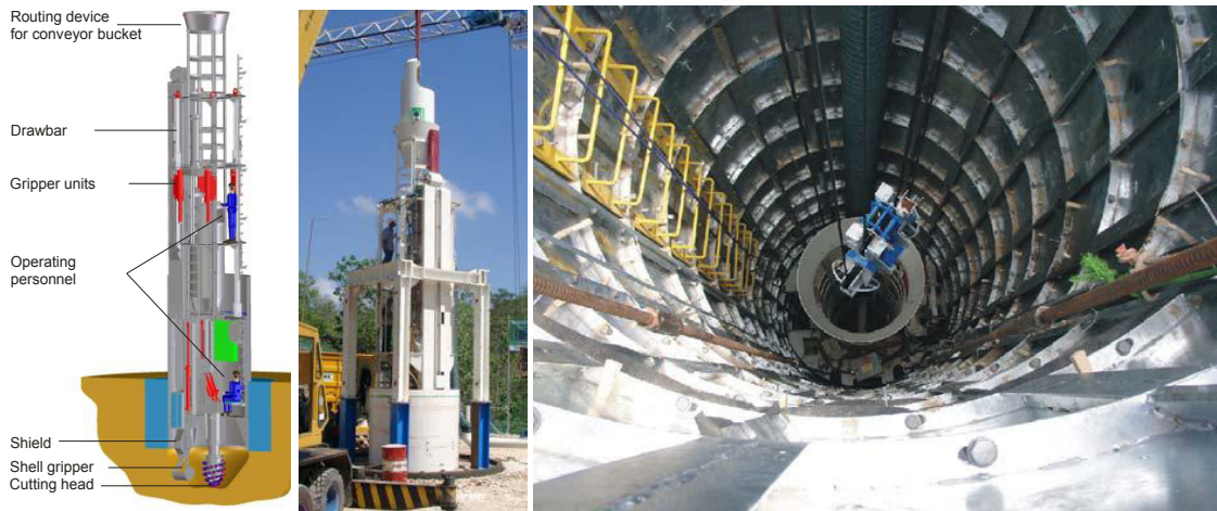
Figure 3. Application of the vertical drilling machine (left) and view into the developed shaft with a depth of 100 m (right)
