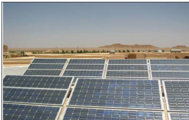
Fig. 1. Photovoltaic generator of 2 kW p installed on roof
