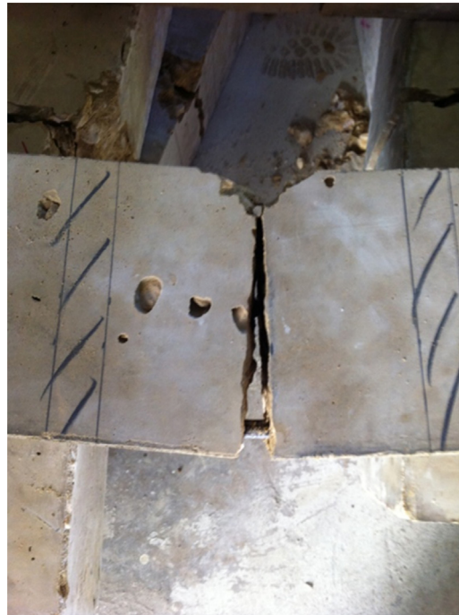
Fig. 10. Failure of a Beam with a Construction Joint.
