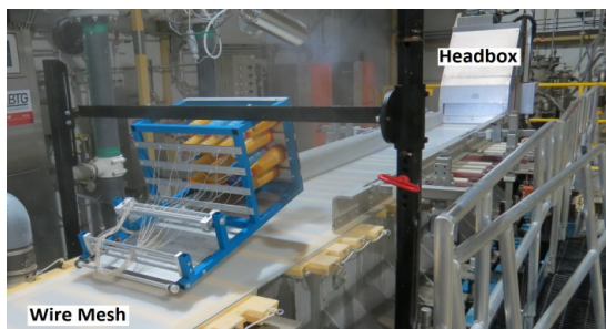
Fig. 4. Installed feeding frame on the paper machine table
