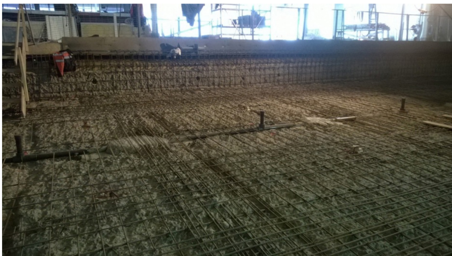
Fig. 5. Upper reinforcement of ground slab. New water treatment pipes were installed before reinforcement.
