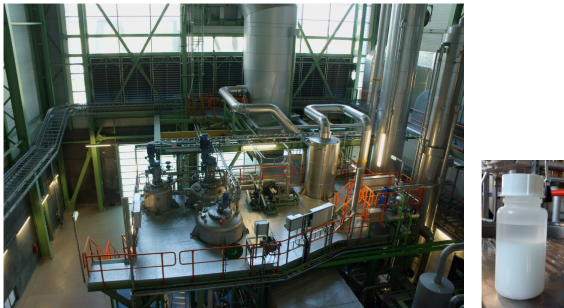
Fig. 5: (a) Overview of the SBC process installed at Twence; (b) picture of first produced NBC slurry
