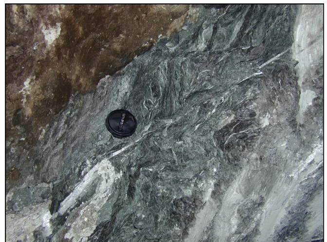
Fig. 5. Tectonically strongly sheared siltstone: a chaotic structure with pockets of clay from a great thrust of different geotectonic units (Anthochori tunnel–Egnatia highway, Northern Greece).
