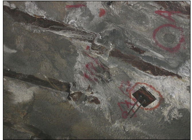
Fig. 8. Overstressed steel sets due to squeezing. Long cables have been implemented to secure stability (Driskos tunnel in Northern Greece).
