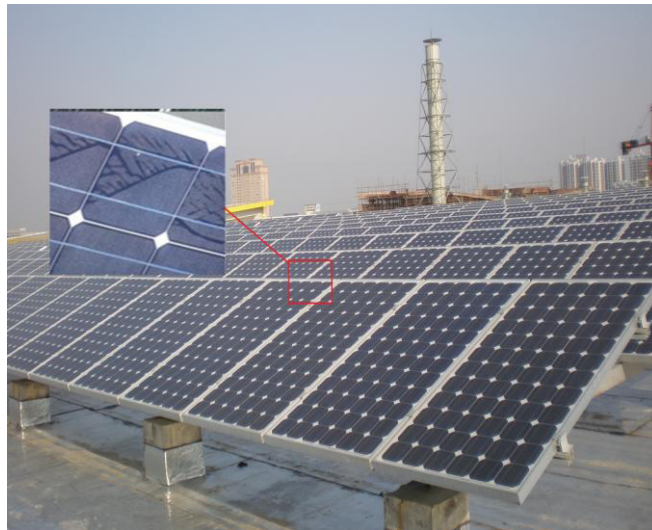
Fig. 1. Phenomenon of snail trails in urban photovoltaic energy systems
