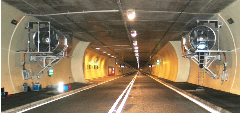
Fig. 6. Example of jet fans for smoke confinement in tunnels with transverse ventilation systems, installation in the Bosruck tunnel, Austria.
