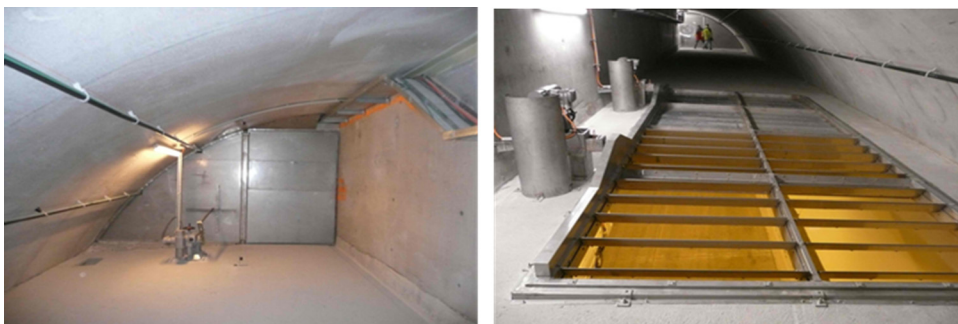
Fig. 8. Example of a motorized damper used for fresh air injection (right), and duct separation wall (left), installation in the Katschberg tunnel, Austria.
