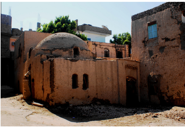
Figure 3 Hassan Fathy's house. The condition of the house has declined dramatically since the architect and the house's janitor passed away. Now the house is deserted and inaccessible [15].
