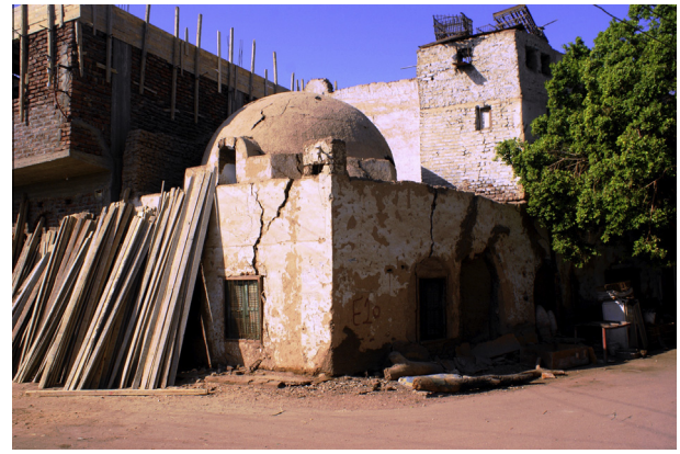
Figure 5 An example of the buildings designed by Hassan Fathy in New Gournia Village that suffer from the spread of deep cracks throughout their earthen walls, and from the dramatic decline in their condition [15].
