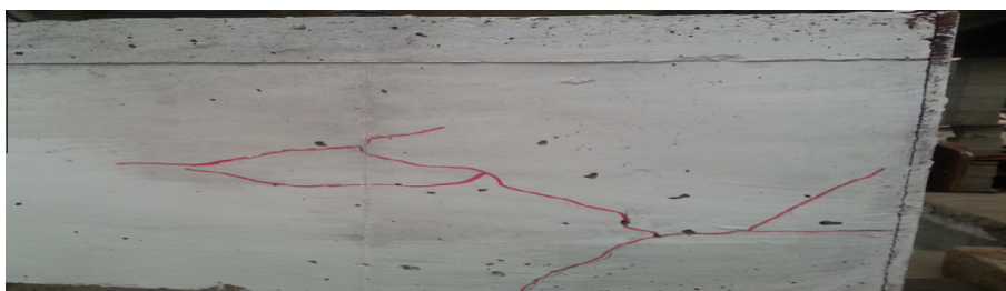
Fig. 14 Hair crack at anchorage zone.
