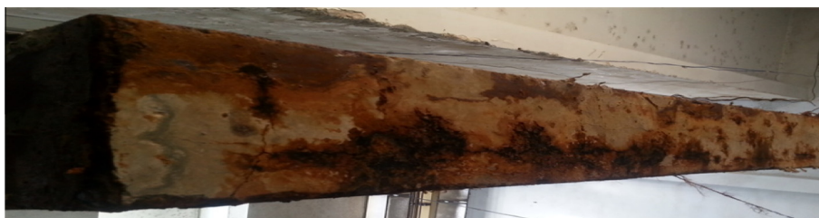
Fig. 13 The deterioration of the concrete against corroded rebar for samples.
