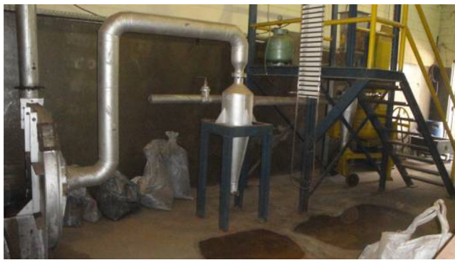
Fig. 1 – Pilot Plant sintering downstream of Metaflexi installed at ArcelorMittal Piracicaba, with exhaust flow capacity 1200 m 3 /h that upon ignition produces a thermal front that reaches 1200 °C, to sustain the heat transfer layer top of the mixture, into the pan sintering, to the bottom layer. Author (2012).
