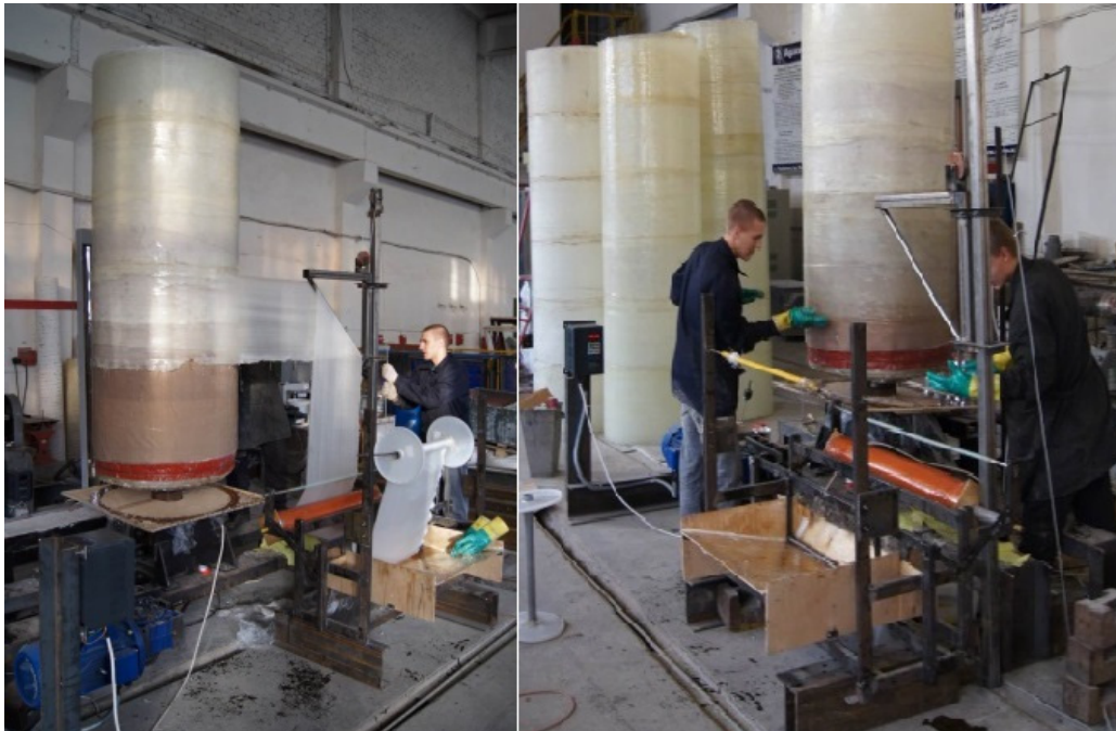
Fig. 3. The installation of vertical winding in the process of work (produced shells in the background)
