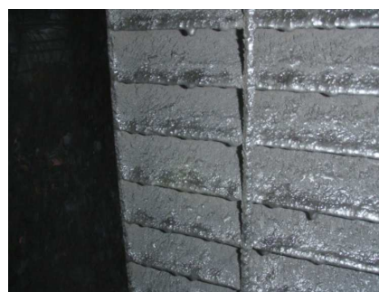
Fig. 11. Dust settled on louvers (Prostański 2012b)
