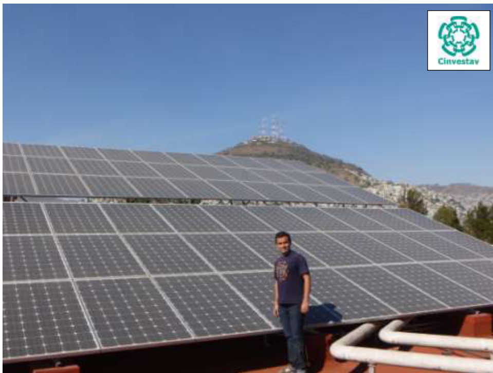
Fig. 1. Part of 60 kWp system PV module array. Each PV module consists of 250 Wp power unit, and total of 240 modules connected to 5 inverters. (Chiquihuite's mountain can be seen at the North direction at the back; 2730 meters high over sea-level)
