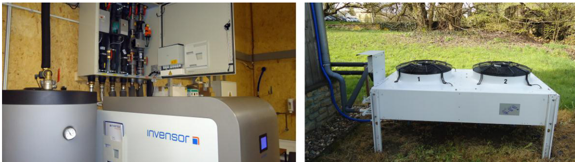
Fig. 2. Solar air-conditioning system pictures; (a) adsorption machine, hydraulics module and hot storage tank; (b) dry cooling tower.
