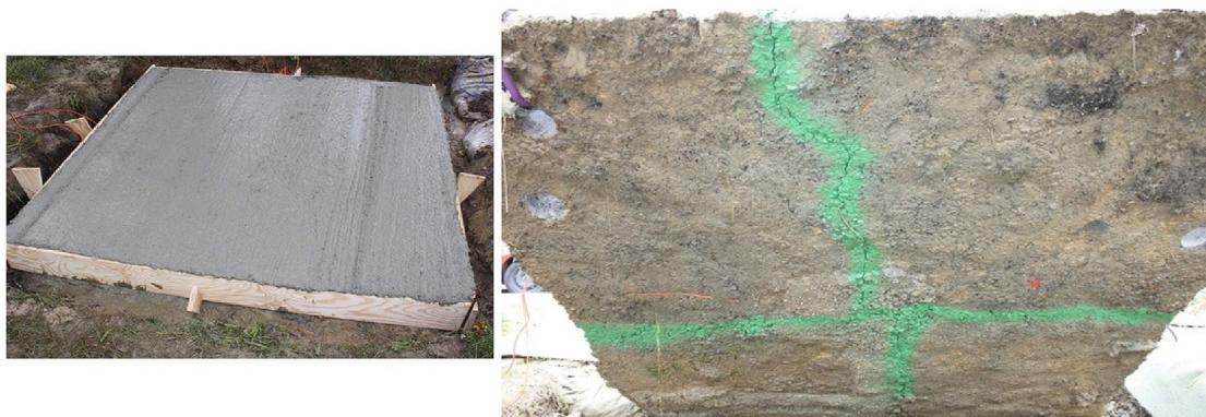
Figure 1 Casting of the steel-fibre reinforced concrete slab and cracks at the lower surface of the failed steel-fibre reinforced concrete slab after its lifting up.
