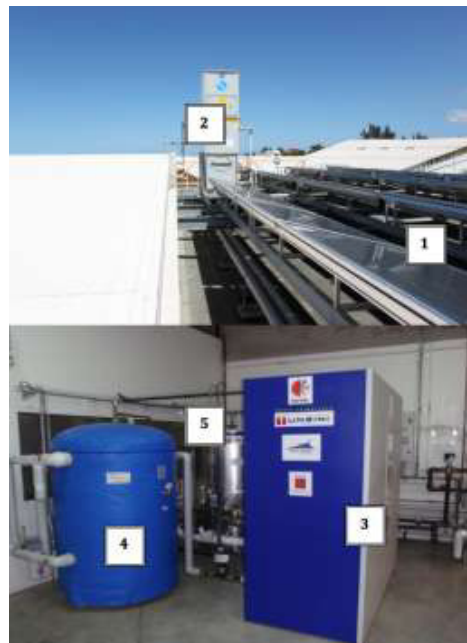
Figure 2b Photographs of the solar absorption cooling system : 1 - Solar collector field ; 2 - Cooling tower; 3 - Absorption chiller ; 4 - Hot water storage tank; 5 - Cold water storage tank
