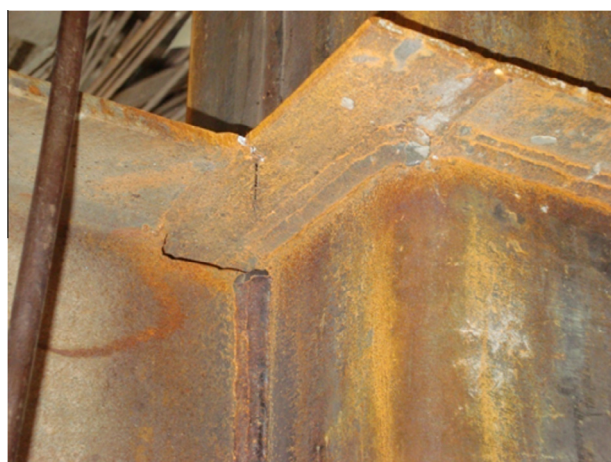
Fig. 9 Stiffener failure for specimen CS-50-6.
