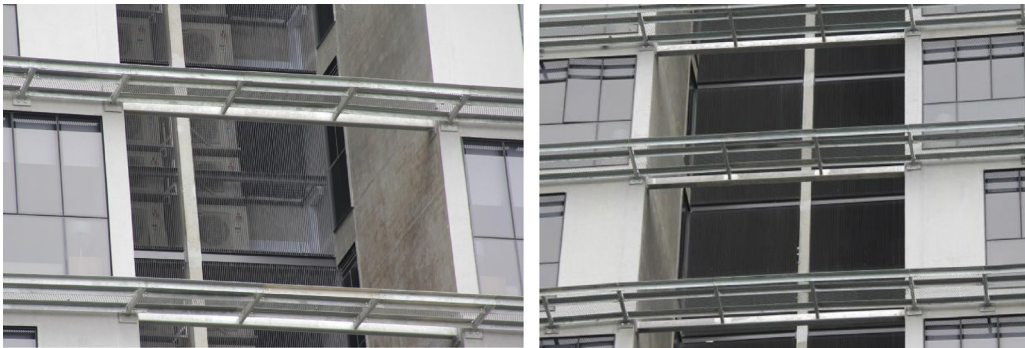
Fig. 3. Condensing units with louvres: split units visible (left) and hidden from view (right).
