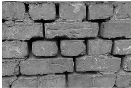
Fig. 5. Extensive loss of mortar in masonry in building C.
