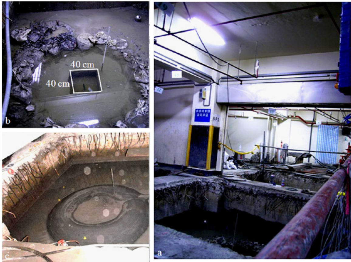
Fig. 4. (a) Photo of a pit near diaphragm wall before sand boiling, (b) a hole left by withdrawing intermediate pile in the pit, and (c) sand boiling in a pit next to the grouting pit.
