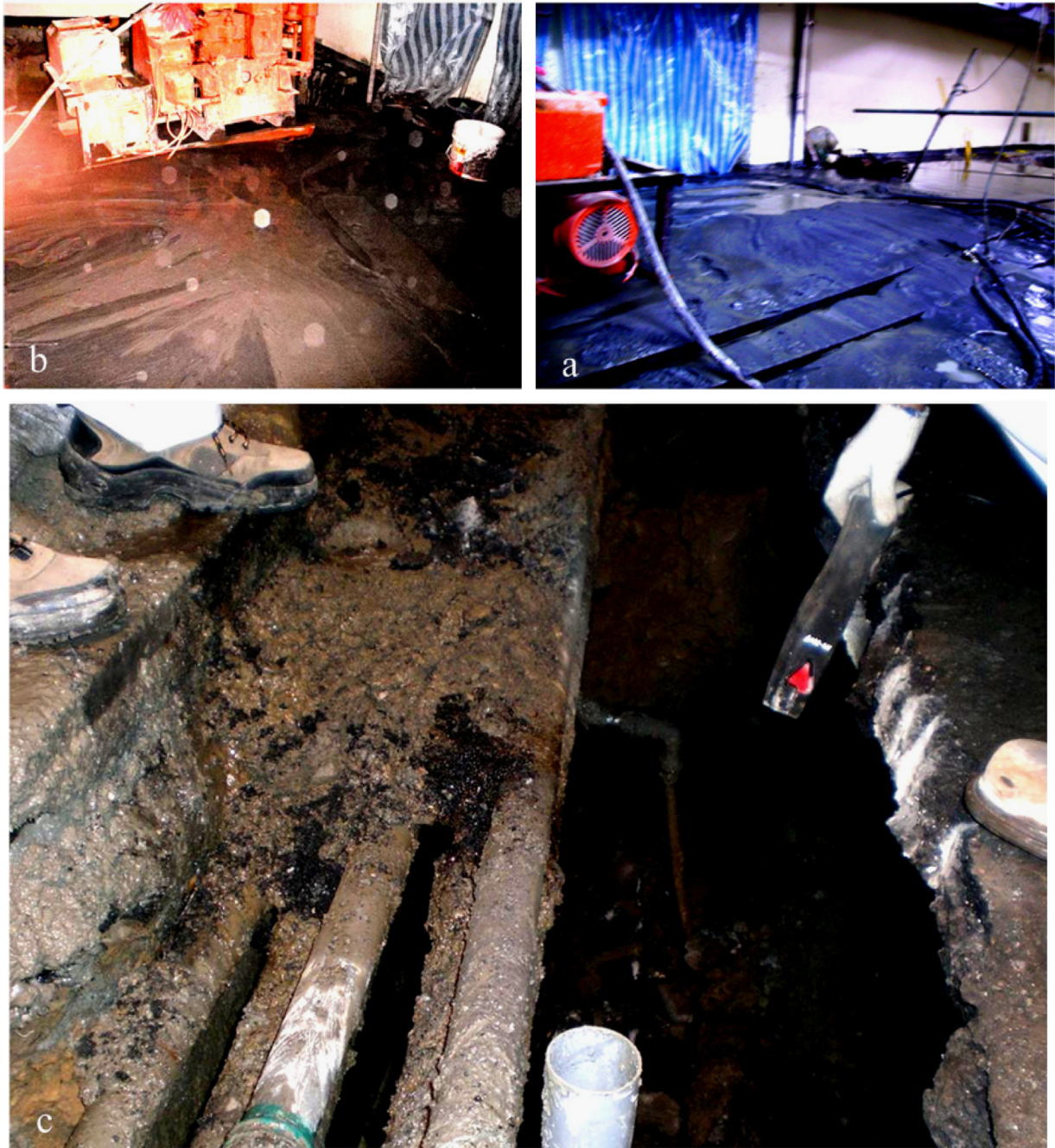
Fig. 5. (a and b) Pits flooded with boiling sand and (c) a surface settled area.
