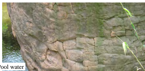
Fig.48 Severely weathered rock surface with blocky cracks exposed above water.
