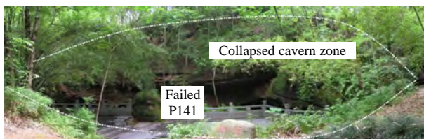
Fig.34 Site photograph showing the collapsed rock cavern No.14 and its water pool.
