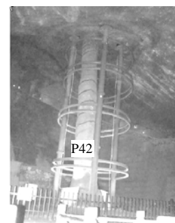
Fig.52 Steel structure supporting measure for rock pillar P42 in the complete rock cavern No.4.
