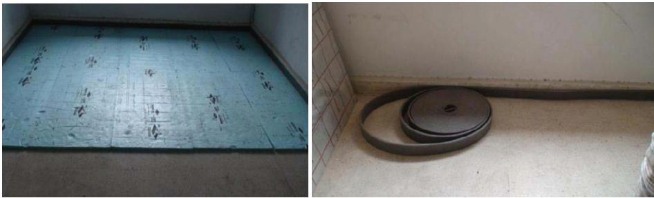
Fig. 4. (a) Thermal Insulation; (b) Surrounding insulators
