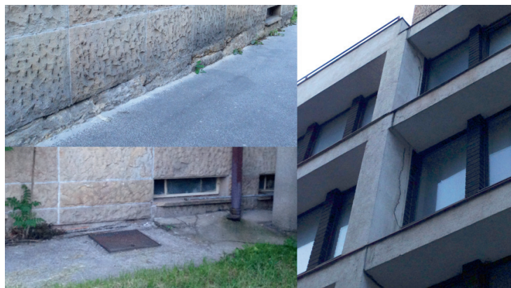
Fig. 4. Photo-documentation of structural deformations over building affected by the construction works on a nearby hotel.
