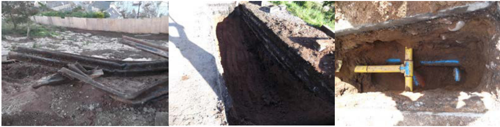
Figure 1. Buried structures and services exposed during construction which were not recorded previously: a) retaining structures b) earthworks c) utility pipes below the recorded gas pipe.
