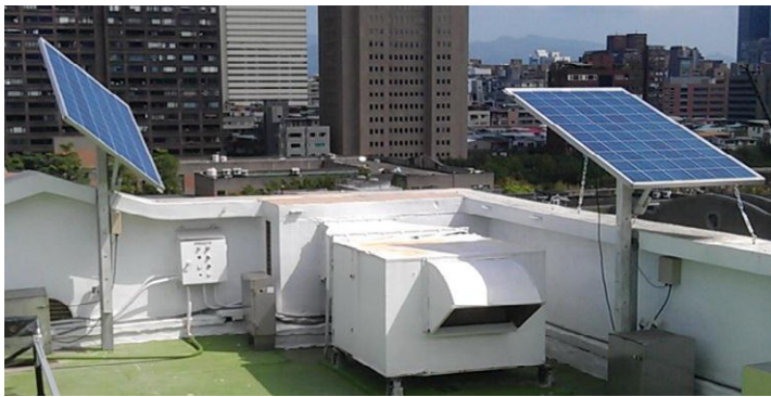
Fig. 1. Comparative test of 1A-3P sun tracking PV.
