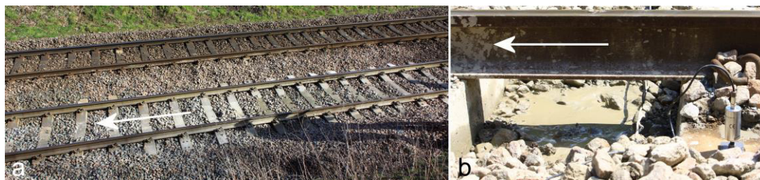
Figure 2: (a) Wet bed prior to track renewal. (b) Close-up of worst region – slurry and pea gravel also visible. Arrows show direction of travel on affected line.
