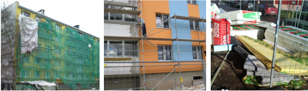
Fig.1. (a) Partly covered scaffolds; (b) Scaffolds without any protection net; (c) Material storage (Liisma et al., 2014).
