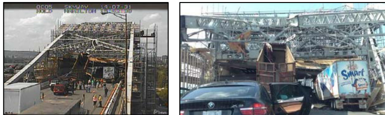
Fig. 1. BrTS, dump truck hit scaffolding after leaving bucket raised on the Burlington Skyway Bridge (Canada), Toronto Sun (2014).
