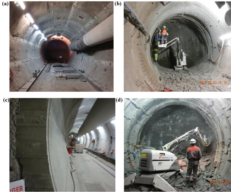
Fig. 3. Example of four different drifts: (a) GCS with compressible concrete wedge, (b) GCR with concrete lining grouted in place, (c) BPE with 0.45 m of shotcrete projected in four layers, (d) GED drift with classical support, shotcrete and sliding steel arches.
