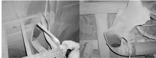
Fig. 1. Pipe rupture due to internal explosion at Hamaoka NPP [2].
